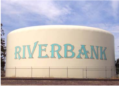
SETTING-17 City Water Tank
